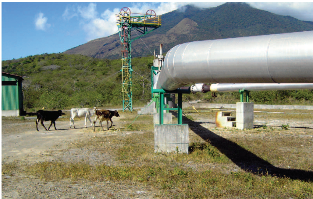
Figure 8.1 Typical pipeline at Miravalles geothermal power plant, Costa Rica (photo by R. DiPippo).
