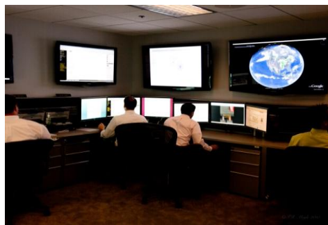
Recovery Operations Center
