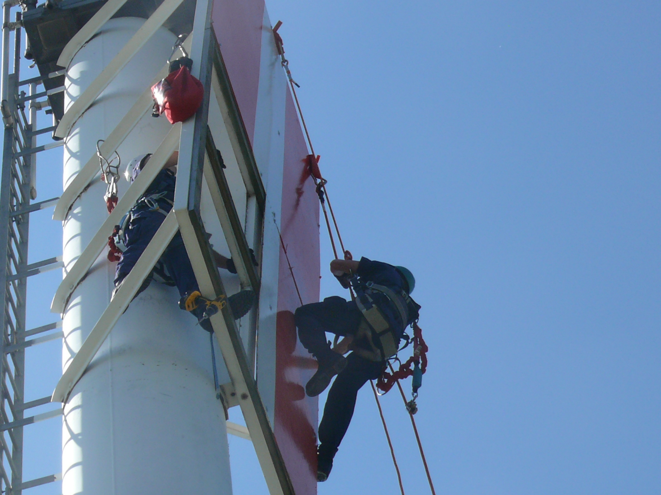
Crew from ANT Detroit and the District Nine Training Team working on Sandusky Range Rear Light. Photo by BM3 Kohl.
