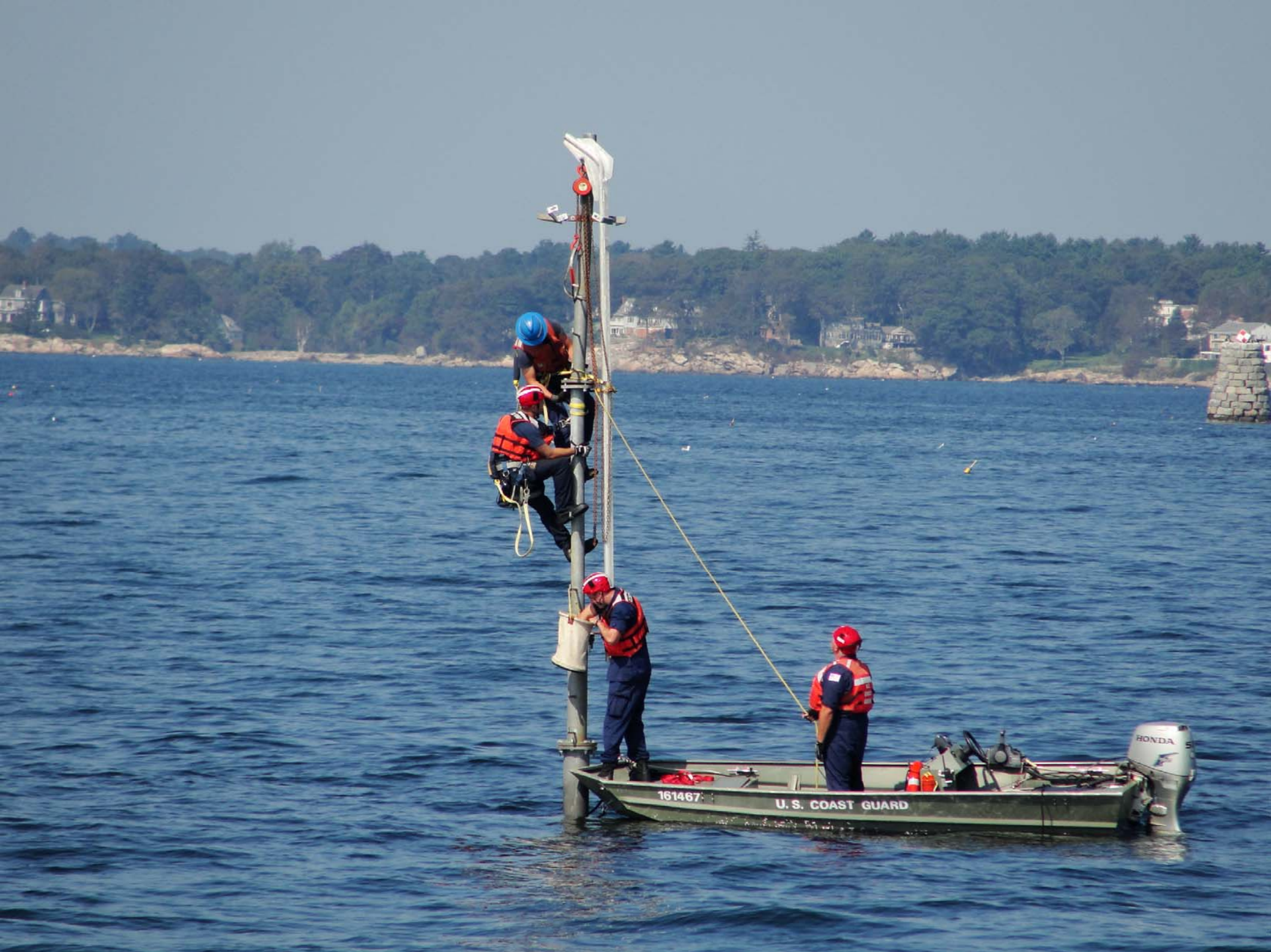
The crew of USCGC PENDANT (65608) working to repair Hardy Rock Daybeacon 1. Photo by BMC Bromwell.
