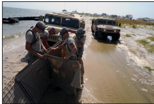
Soldiers of the Alabama National Guard build and maintain miles of HESCO barriers to protect Dauphin Island, Ala., beaches from the BP oil spill, July 23, 2010.
