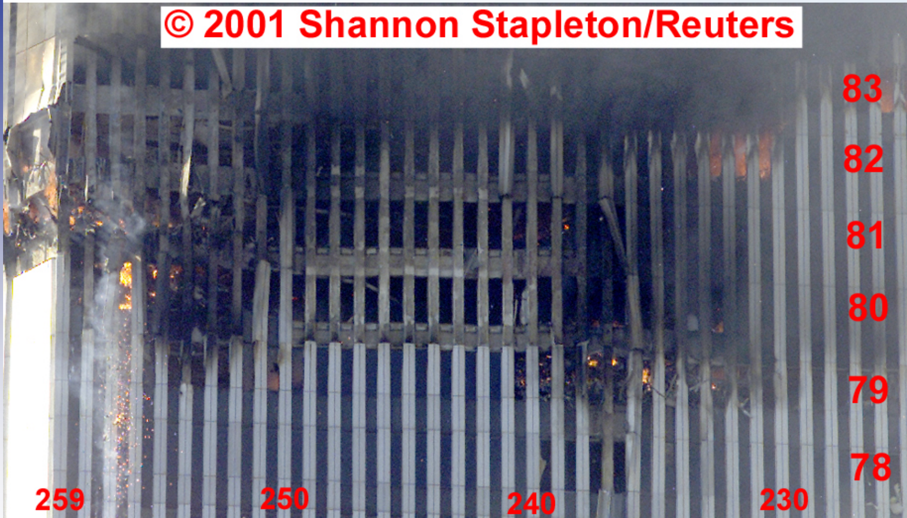
North Face of the South Tower. Image shows what appear to be portions of several floor slabs hanging across window openings on Floors 80, 81, and 82
