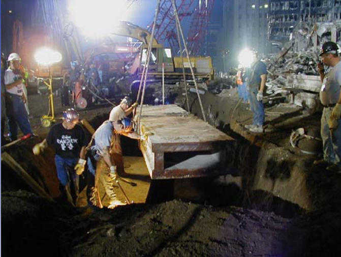
Clean weld fracture of Interior columns
