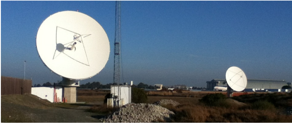
Figure 4. Antennas at Ames Research Center
