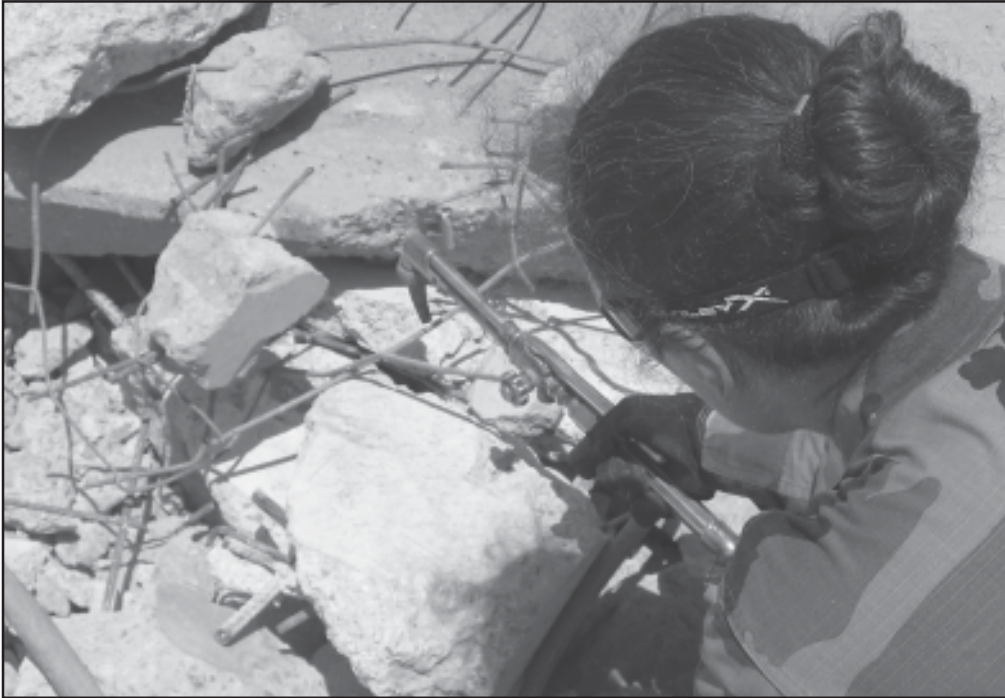
Capt. Sampsonis learns to use a blow torch to remove reinforced steel from an entry way.
