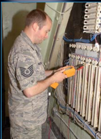
Tech. Sgt. Joe Richardson uses a telephone test set to troubleshoot and verify that specific phone circuits are working correctly.
