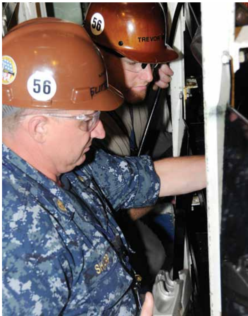
▲ Onboard USS Memphis, Surgemain reservist Chief Machinist Mate Scott Sharp and Shop Pipefitter Trevor Watt work with a Lokring machine which places caps on hydraulic lines.
