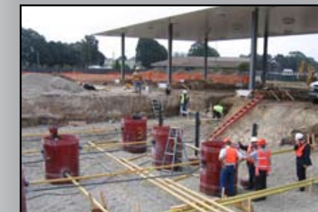
Air Force contractors review progress of the fuel station project at Vandenberg AFB, California.
