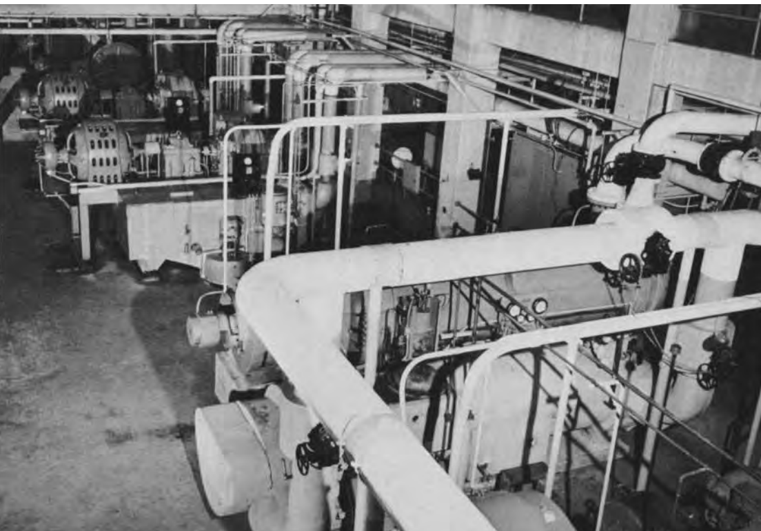
Central refrigeration and air conditioning machinery—Power Section.
