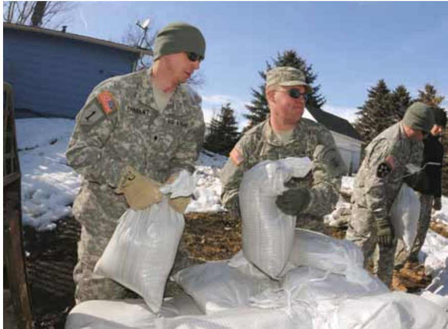
SPC Tim Sybrant of the 817th Engineer Sapper Company, left, and PFC Scott Ness of the 188th Engineer Company build a sandbag flood barrier to hold back rising water from the Sheyenne River.
