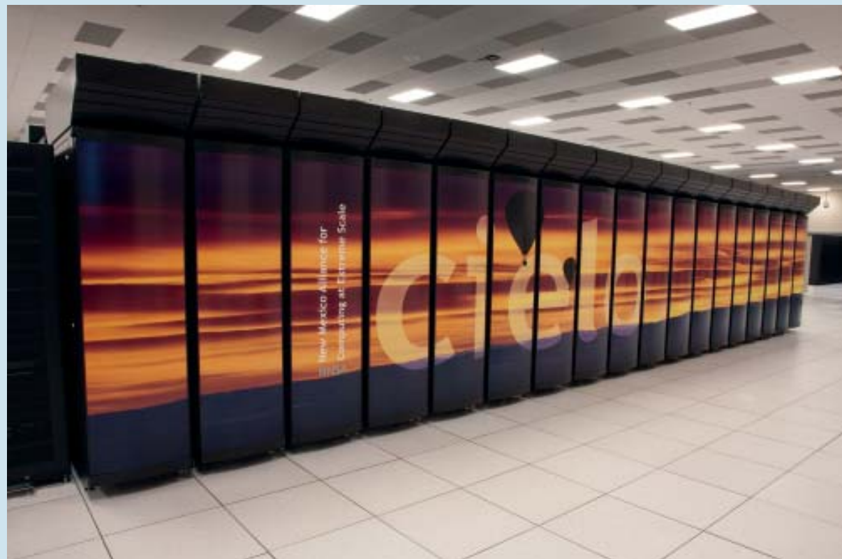
PREDICTIVE CAPABILITY: Housed at Los Alamos National Laboratory, NNSA's petascale supercomputer Cielo runs the largest and most demanding workloads involving modeling and simulation.
