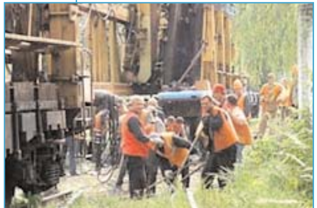
Russian crews remove track at the entrance to a Ministry of Defense Facility near the City of Bryansk, Russia. A Volpe team examined rail construction and inspected missile launch cars destined for elimination at this facility. (Photo courtesy of Mr. Ross Gill)
