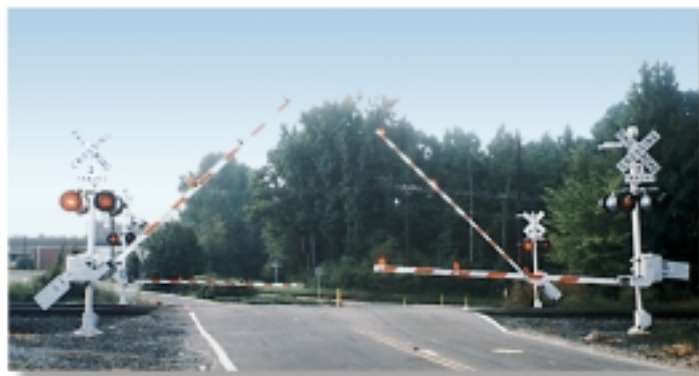
Four-quadrant gate systems are sometimes used with a median barrier to further deter violations.
