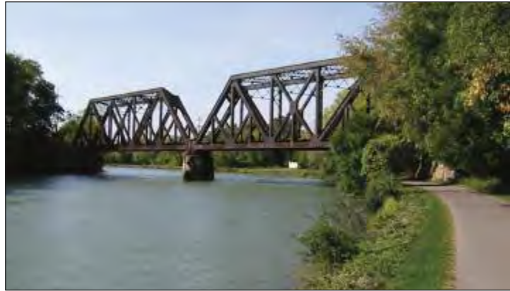
A trespass detection and deterrent system installed on a railroad bridge in Pittsford, New York. This equipment allows railroad security to remotely monitor ROW and respond to incidents effectively.
