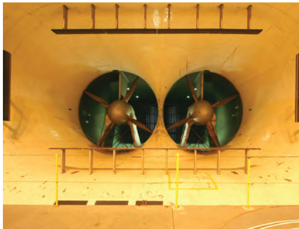
Current view of fan blades.
