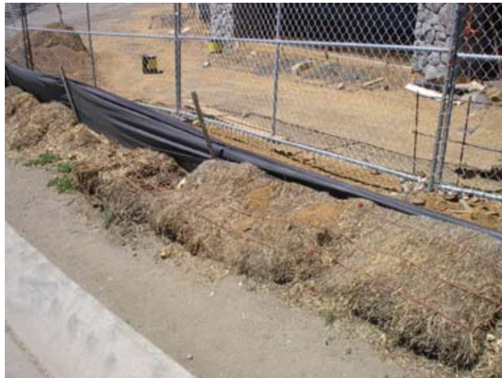
Photo 2: Hay bales and silt fence that are in need of maintenance
