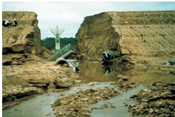
Figure 5-4 Leakage through a defective joint in a corrugated metal pipe outlet works conduit (FEMA, 2005)
