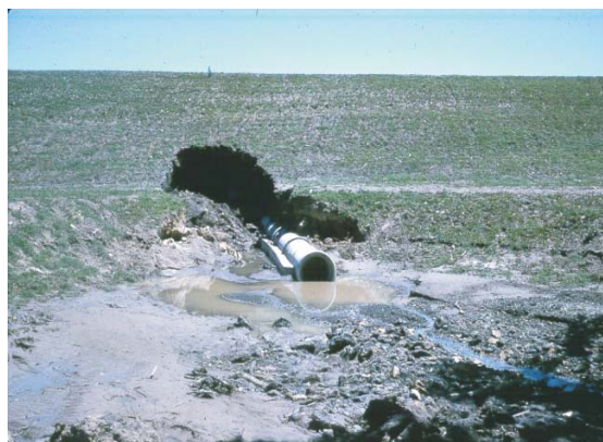
Figure 5-2 A failure due to internal erosion often leaves a tunnel-shaped void along the conduit (FEMA, 2005)
