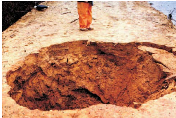
Figure 5-1 Sinkhole which developed over Spillway Conduit (FEMA, 2005)
