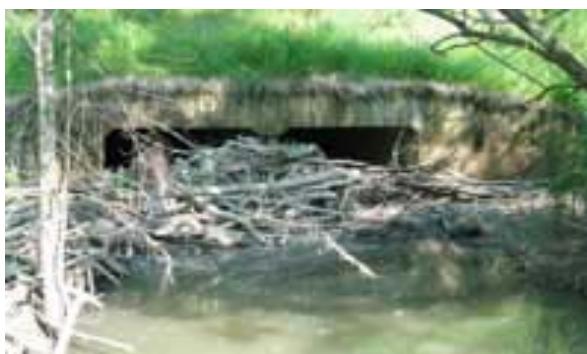
Figure 5-12 Upstream Debris on Dam Outlet (Rizzo Photo, 2007)
