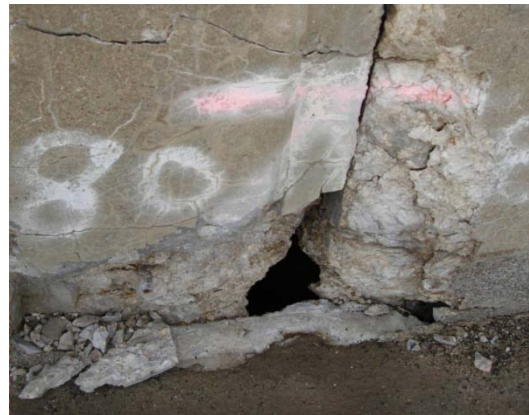
Figure 5-15 Surface Cracking - Alkali-Aggregate Expansion (Rizzo Photo, 2007)
