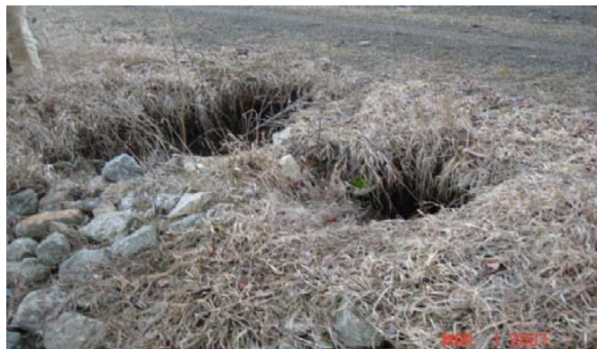
Figure 5-6 Embankment Sinkholes (Rizzo Photo, 2007)
