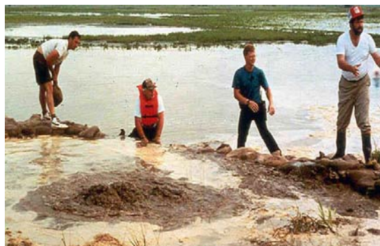
Figure 5-9 Embankment Seepage Advanced (Rizzo Photo, 2007)
