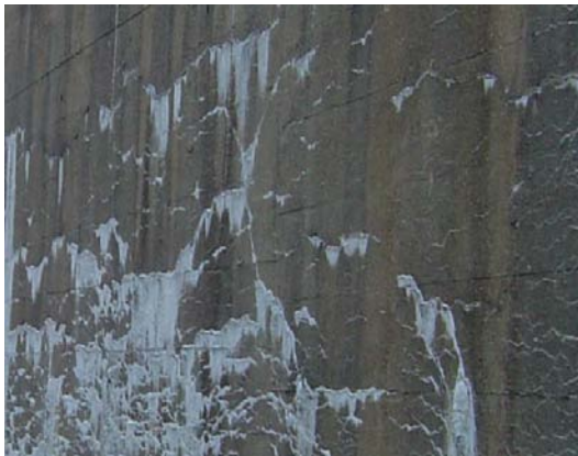
Figure 5-16 Structural Crack Monitoring (Rizzo Photo, 2007)
