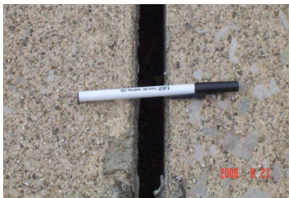
Figure 5-19 Displacement of Joints (Rizzo Photo, 2007)
