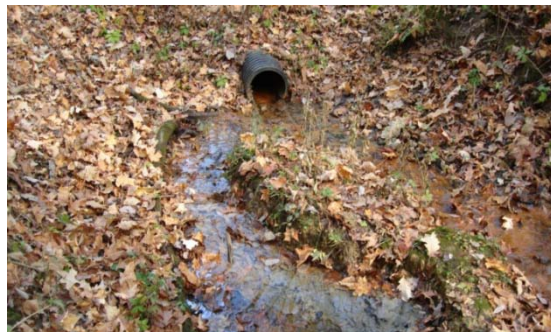
Figure 5-8 Embankment Seepage (Rizzo Photo, 2007)
