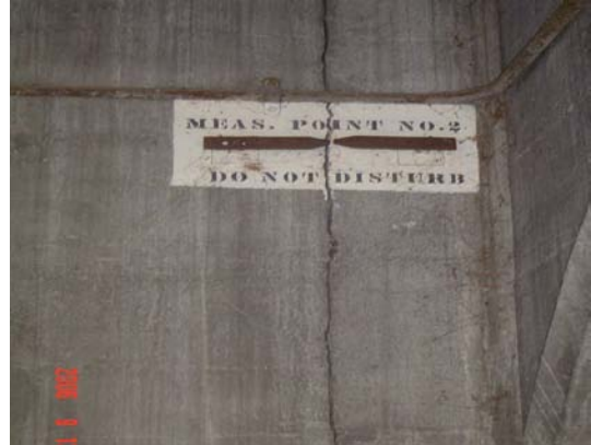
Figure 5-14 Structural Crack (Rizzo Photo, 2007)
