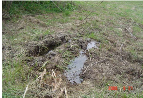
Figure 5-7 Embankment Seepage (Rizzo Photo, 2007)
