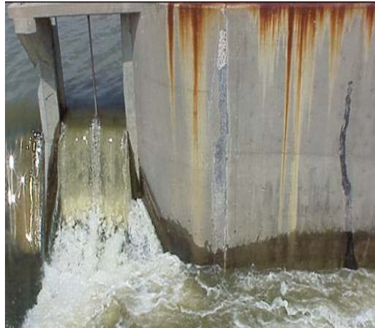
Figure 5-17 Spalling (Rizzo Photo, 2007)
