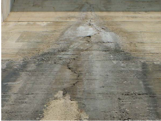
Figure 5-13 Structural Crack Monitoring (Rizzo Photo, 2007)
