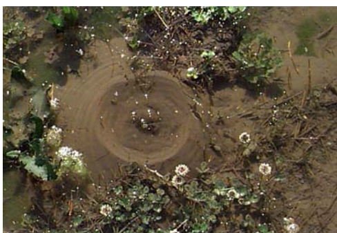
Figure 5-10 Embankment Sand Boil, Early State Piping (Rizzo photo, 2007)
