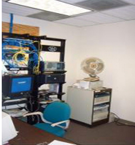
Figure 5: ICE server not secured in a locked cabinet
