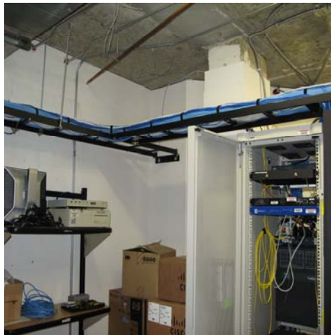
Figure 6: TSA server room used for storage
