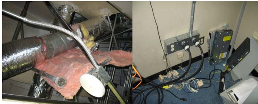
Figure 2: Missing ceiling tiles and inadequate storage at LAX.
