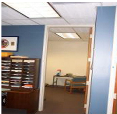
Figure 4: ICE server room with open door
