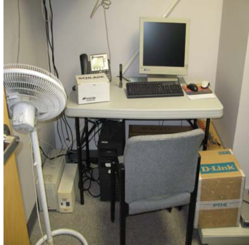
Figure 7: Portable fan used to cool switch and server area
