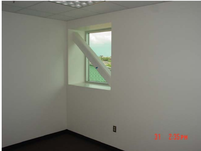
Figure 1. Example of an Improperly Placed Construction Beam
