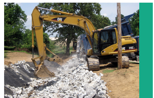
A contractor completes work on a streambank stabilization project in Lynn, Ark.
