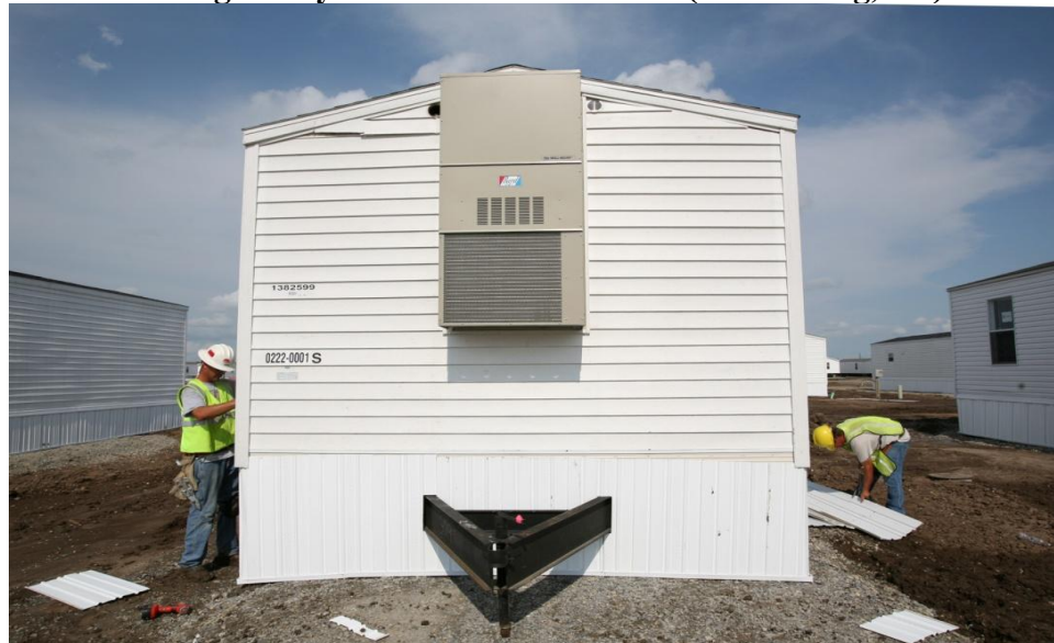
Figure 3. Construction of a temporary housing unit at a FEMA housing site by IA-TAC II contractors (Greensberg, KS)
