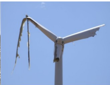
EF1 damage to a wind turbine about 5 miles SE of Spivey, KS
