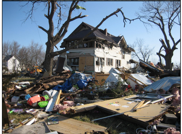
A strong tornado impacted Harveyville, Kansas on the night of February 28, causing significant damage to the town. Photos from NWS storm survey
