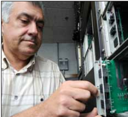
Mr. Eduardo Silva, electronic technician, replaces a fuse card on the high frequency communication system at Lajes Field Oct. 15, 2010. HF communication system is part of a worldwide network of 13 high-power ground radio stations.
