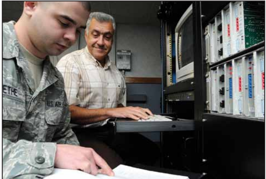
Airman 1st Class Steven Grethe, 65th Communications Squadron transmission systems journeyman, and Mr. Eduardo Silva, 65 CS electronic technician, review the technical order while doing daily checks on the high frequency communications system at Lajes Field Oct. 15, 2010. The high frequency communication system allows the president, vice-president, cabinet members, and other senior government and military officials to communicate in the mid-Atlantic area for command and control while aboard Special Air Mission aircraft. Daily checks are done to ensure that the system transmits and receives information properly. (Photos by Tech. Sgt. Chyrece Campbell)
