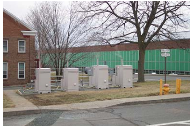
PEM fuel cells operating at Watervliet Arsenal, NY (FEB 02)
