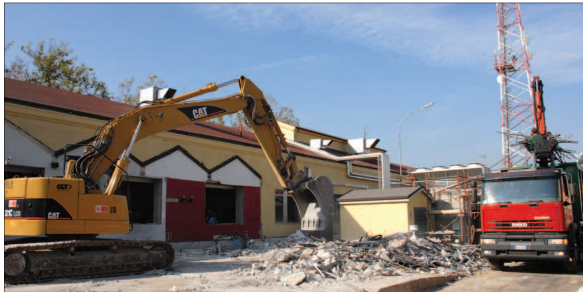
Demolition has already begun on the new construction site for the South of the Alps Dining Facility. This area used to be the Regimental Dining Room. All Soldiers, not just meal card holders, can again use the DFAC under expanded operating procedures starting Oct. 15. (Photo by Gary L. Kieffer, Outlook Staff)
