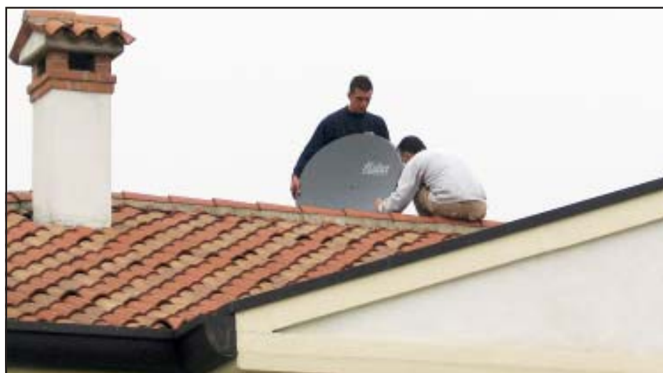
Diego Facin (left) and Luciano Luccarda install the satellite dish on top of a customer's home. The home already had an antenna installed, and the contractors left it in place so the customer will continue to receive reception through the antenna if they wish.
