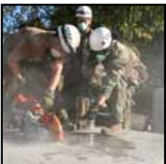
PORTLAND INTERNATIONAL AIRPORT, Ore. - Staff Sgt. Derrick Brooks and Senior Airman Mark McHugh, 304th Rescue Squadron pararescuemen, and 2nd Lt. Michael Vanzanten, a combat rescue officer here, cut a slab of concrete as part of the ROCO Rescue Tactical Confined Space and Collapsed Structure Technician training exercise. (U.S. Air Force photo/Master Sgt. Ruby Zarzyczny)
