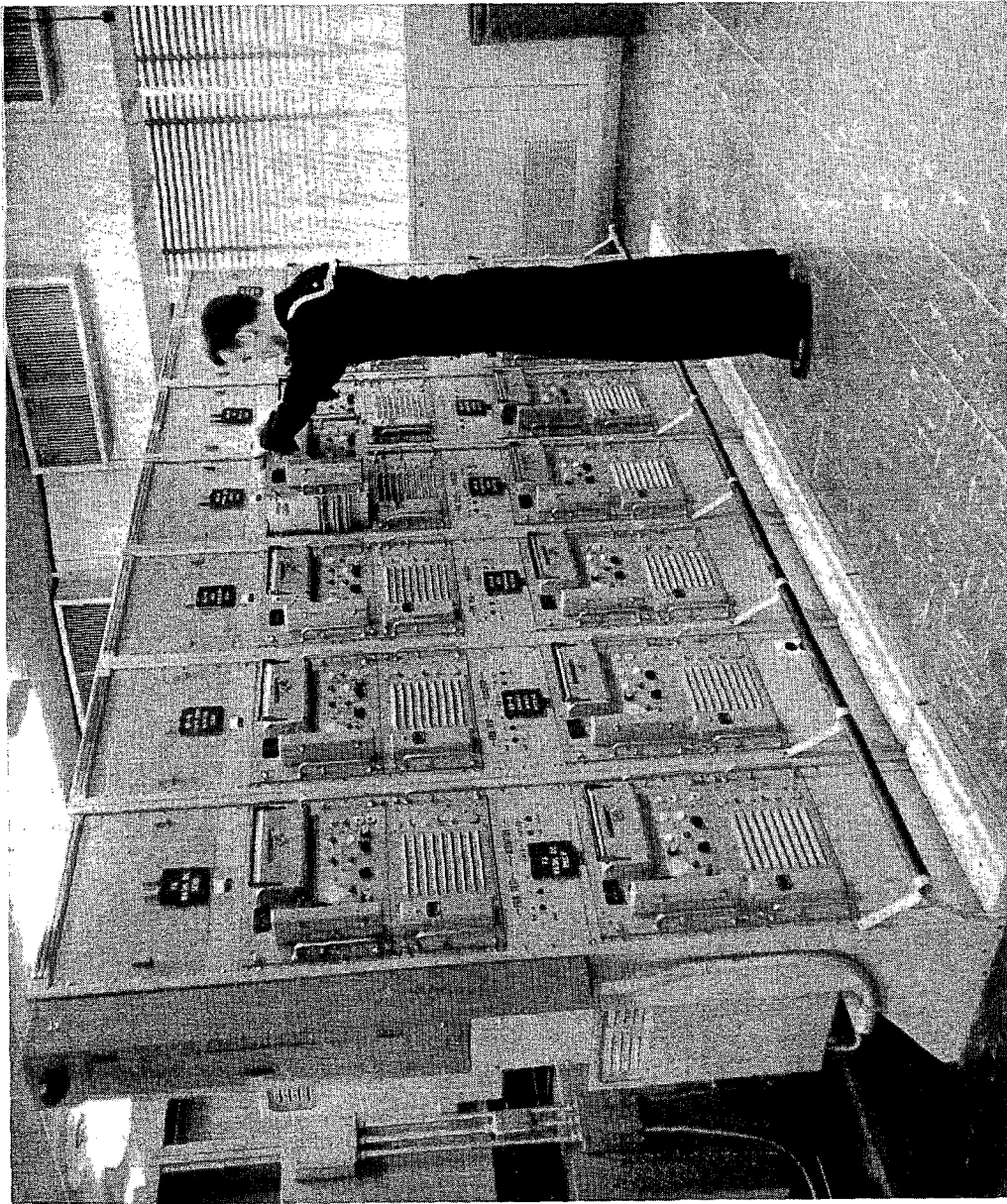
A bank of KW-26s installed in NSA's communications center
