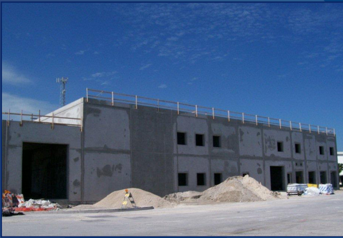
A 10,000-square-foot building is under construction at Coast Guard Sector Key West, Fla., to meet maintenance, storage and personnel requirements for the new Fast Response Cutters that will be homeported there. U.S. Coast Guard photo.
