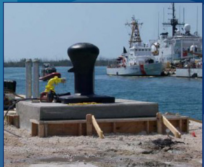
A new mooring bollard is part of the upgrades made to the pier at Coast Guard Sector Key West, Fla., to accommodate new Fast Response Cutters. U.S. Coast Guard photo.
