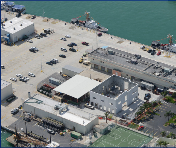
A 10,000-square-foot support building at Coast Guard Sector Miami is under construction in anticipation of the six new 154-foot Fast Response Cutters that will be homeported there. U.S. Coast Guard photo.
