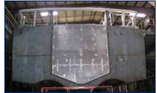
The first FRC is under construction at Bollinger Shipyards in Lockport, La. Shown here is the stern ramp that can launch a small boat to be used as a transport for law enforcement boarding or rescue and assistance teams. U.S. Coast Guard photo courtesy of the Project Resident Office Lockport
