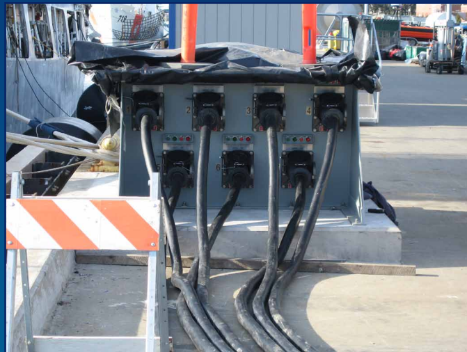
Upgraded electrical shore ties in Alameda, Calif., provide sufficient electrical power at the pier for the modernized systems onboard NSCs. U.S. Coast Guard photo.
