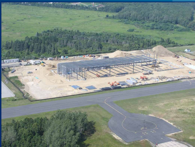
Structural steel is set for the new hangar at Air Station Cape Cod, Mass., which will house HC-144A aircraft. Construction of the hangar is about 25 percent complete. U.S. Coast Guard photo.
