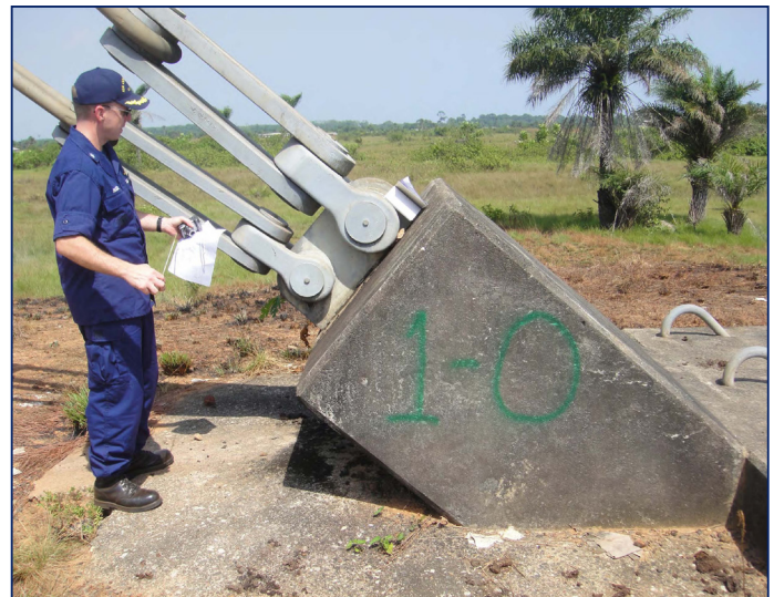
Cmdr. Michael Hudson takes field measurements of one of the tower’s structural guy anchors during a preliminary site visit in April. Photo courtesy of Mark Loiseaux, president of Controlled Demolition Inc.
