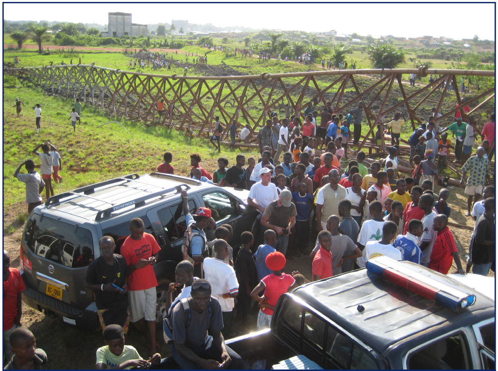
The fallen tower is surrounded by a crowd of Liberians who are overjoyed that the tower has come down safely and will be replaced by a new marketplace. Photo courtesy of U.S. Army Lt. Col. Clement Ketchum with the U.S. Embassy Monrovia.
