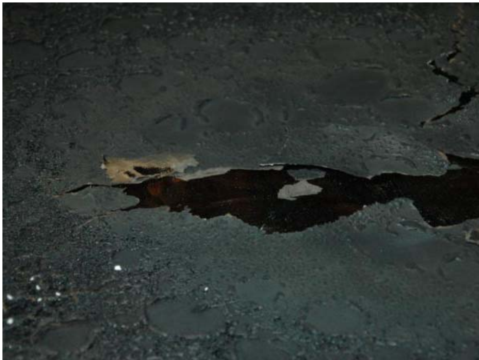
(b) – Degradation of Vinyl due to Kerosene Spill
