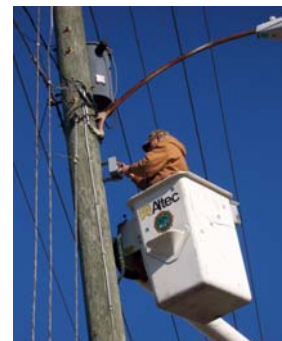
Figure 9: Typical Sensor Installation
