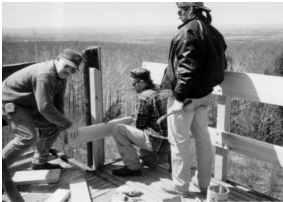
Clients build a lookout tower in a Connecticut state park, which will be used to spot forest fires.
