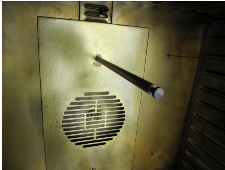
Figure 3: Hanging Rod Installed Above Fan in Oven
