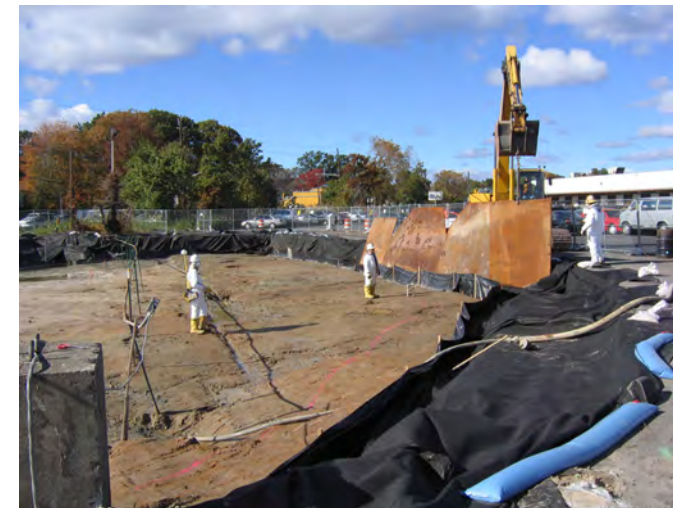
Radiation technicians provide support during the removal of sheet pile used at this Maywood, N.J., vicinity property.
