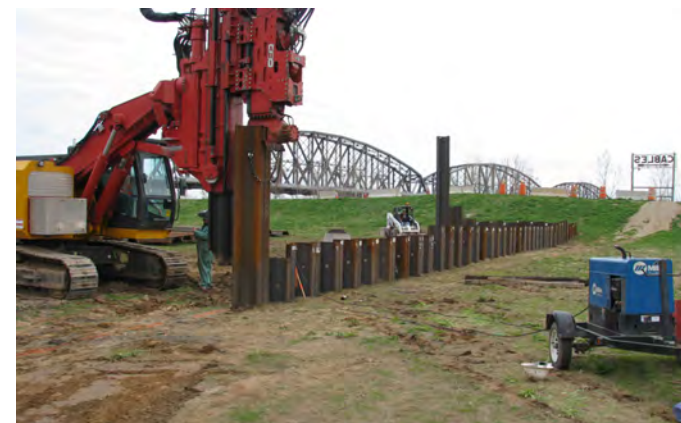
Heavy pile-driving equipment initiates the sheet pile protection for the St. Louis City Vicinity Property at the St. Louis Downtown Site location.
