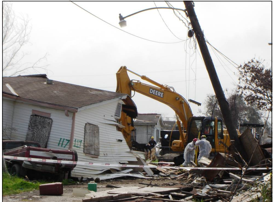
A Corps of Engineers' LA-RFO contract team demolishes a house in New Orleans in September, 2006. The LA-RFO has so far overseen about 3,900 demolitions, over 1,400 demolitions in Orleans Parish alone. (USACE Photo)
