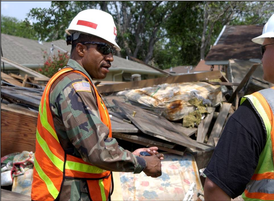
Master Sgt. Gregory Holmes, left, discusses debris procedures with a contractor on the site of an LA-RFO demolition. (USACE Photo)
