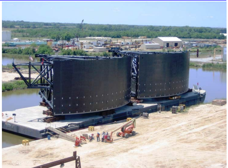
Manufactured by Shaw Global in Delcambre, La., the Inner Harbor Navigation Canal Surge Barrier sector gates are readied for transport to New Orleans. These are the largest of three gated structures in the project. USACE Photo
