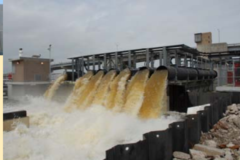
Harvey Canal Floodgate & Pumps
