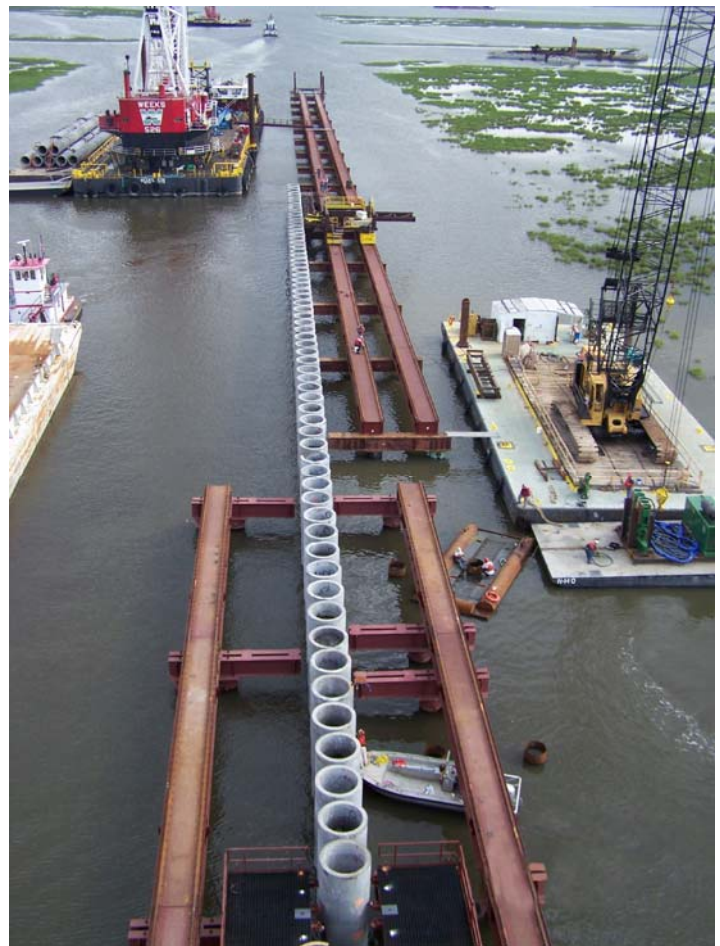
The Corps is working around the clock to build the IHNC Surge Barrier. On June 2 crews had 624 linear feet of spun concrete piles in place. When completed, the barrier will be 10,000 feet wide with 3 navigable gates. (USACE Photo)
