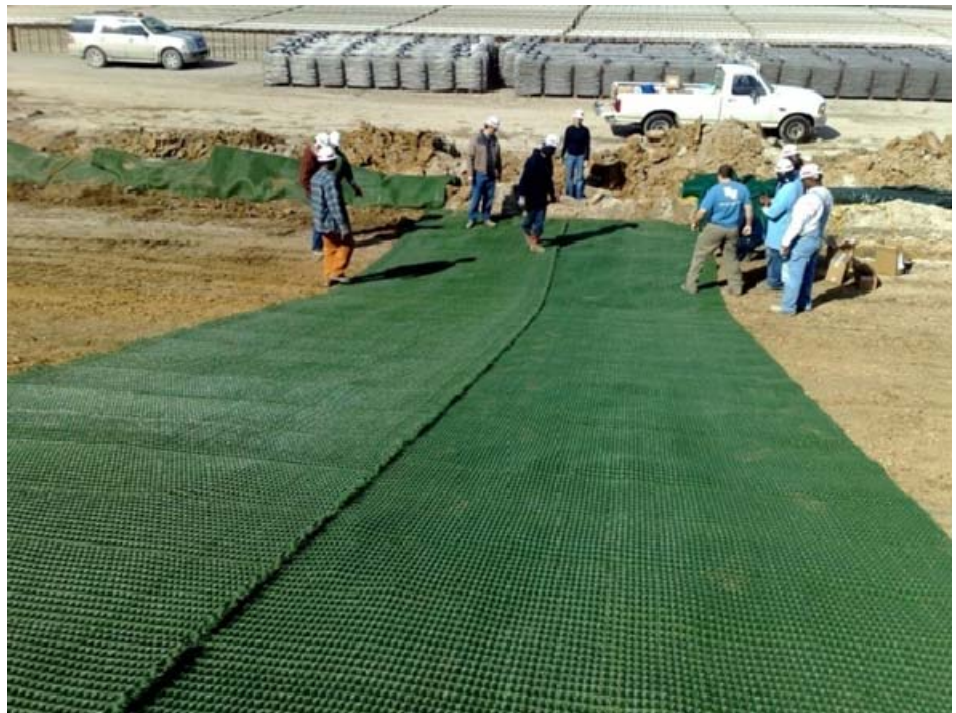
Crews install Turf Reinforcement Mats on a levee. The TRM will further strengthen the levee in the event of overtopping.
