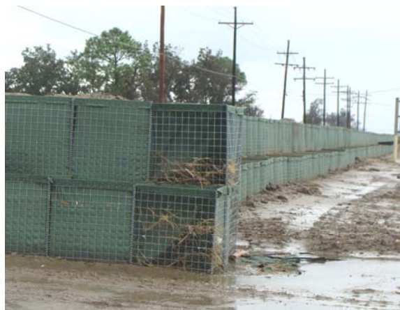
Hesco baskets are wire and fabric containers that are filled with sand or gravel to temporarily close a construction opening or gap during storms.
