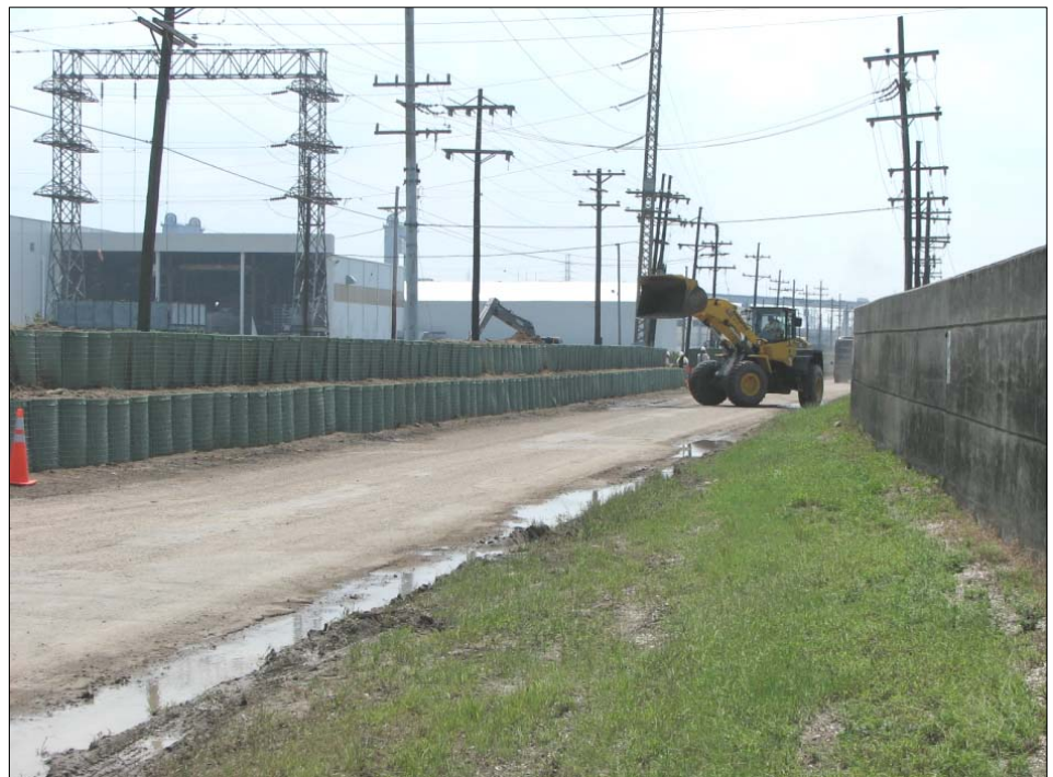
In advance of an expected tropical event, the Corps will often use Hesco baskets to temporarily close openings or gaps in the system where construction is incomplete. Prior to Hurricane Gustav in 2008, the Corps placed sand-filled Hesco baskets (above) along the Inner Harbor Navigation Canal west wall. USACE Photo
