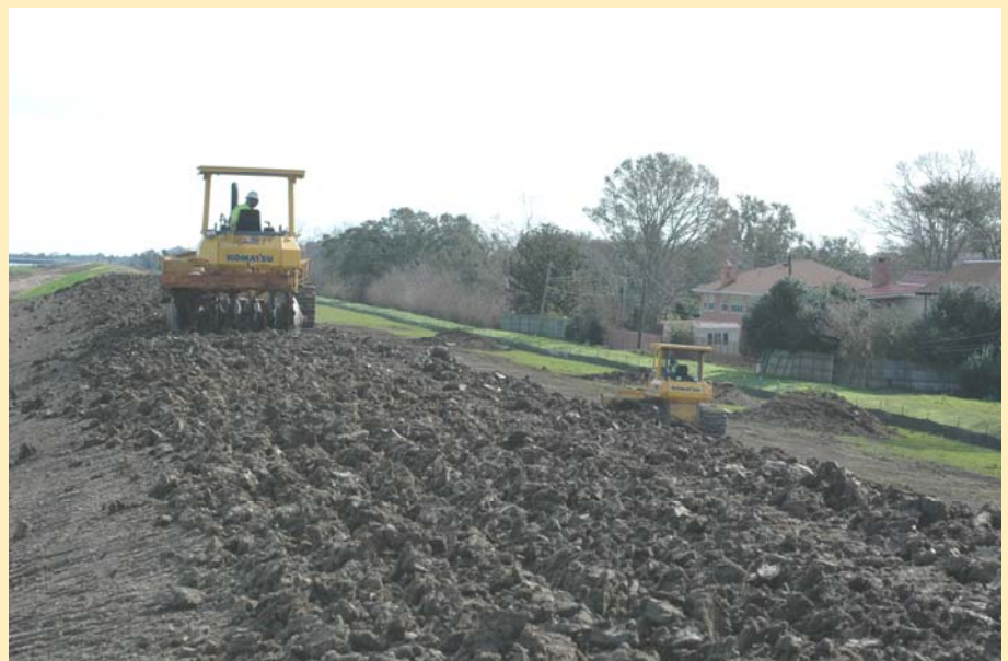
Bulldozers scarify a levee surface to prepare it for a new levee lift.
