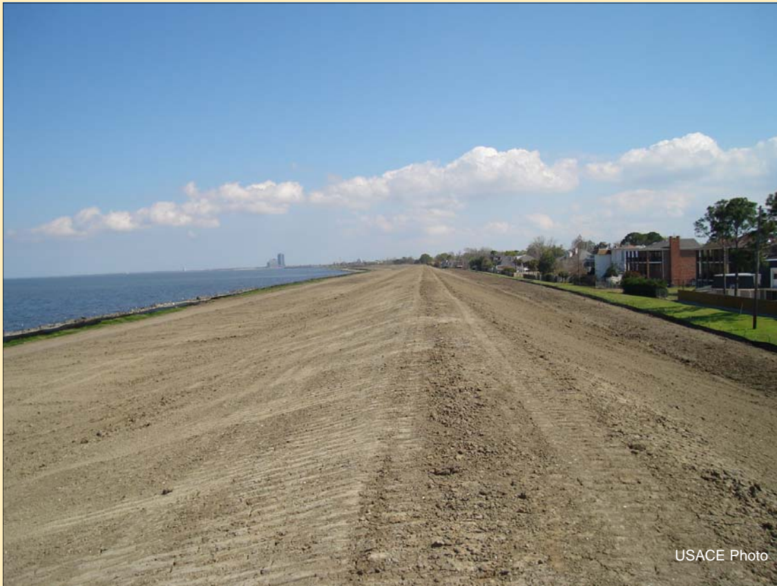
This levee section has recently been lifted to meet the 100-year criteria.
