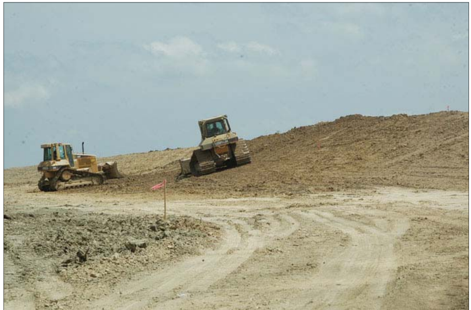
Bulldozers push soil material up an earthen levee to build a new levee lift. Future levee lifts along the HSDRRS will be needed to maintain the authorized level of risk reduction. (USACE Photos)
