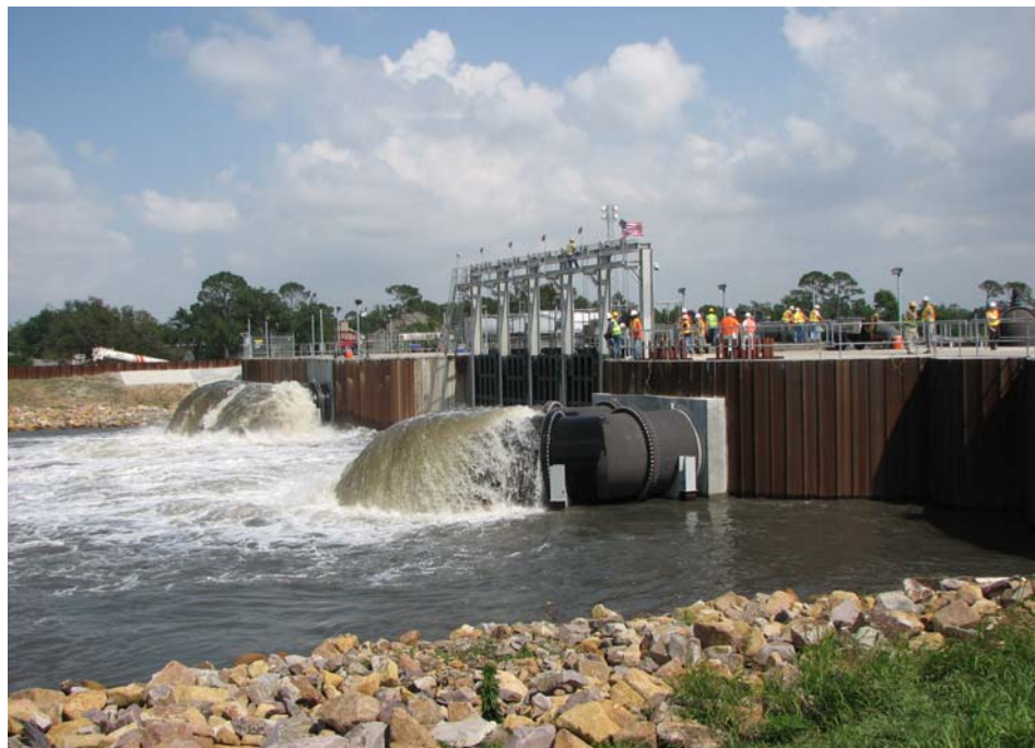
Corps of Engineers employees perform a pump test at the Orleans Ave. Outfall Canal. Tests are performed on a regular basis on all pumps, pump station equipment, gates and flood fighting equipment to ensure everything will be ready for a possible tropical event.
