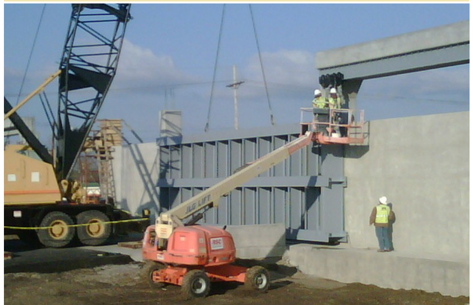
The Highway 46 gate on the northbound lane in St. Bernard Parish is one of 499 openings in the HSDRRS that will be closed to halt storm surge prior to a hurricane reaching the area .
