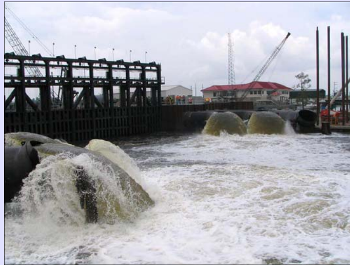
17th Street Outfall Canal pumps and gates perform during recent test.
