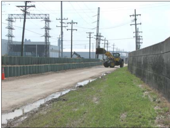
TOP: HESCO baskets are placed at the IHNC west wall prior to Gustav to reduce risk of flooding.
