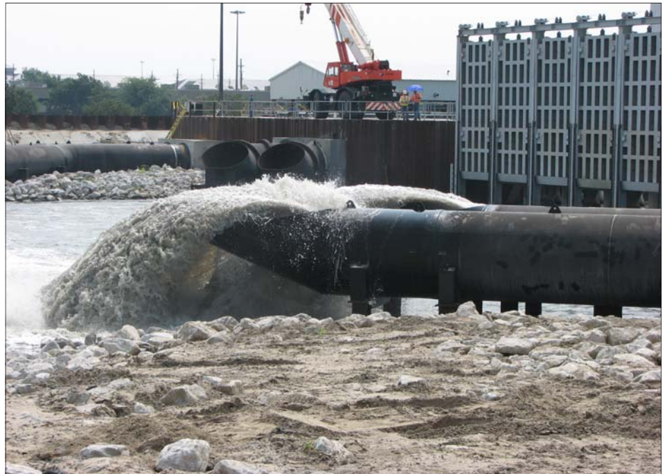
The London Ave. Outfall Canal pumps and gates (shown above during a recent exercise) and the 17th Street Outfall Canal pumps and gates were put to the test by Hurricane Gustav on Sept. 1. Both structures performed as designed and allowed the Sewerage & Water Board to run its pumping stations. (USACE Photo)
