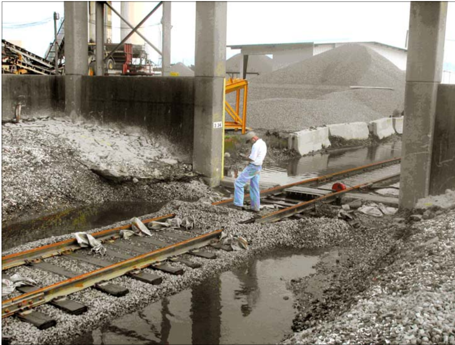
A Corps technician inspects a railroad gate along the HSDRRS that had some damage during Hurricane Gustav. (USACE Photos)
