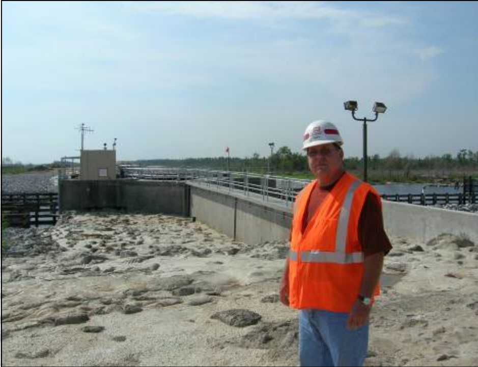
Steve Falati, a Construction Representative for the New Orleans District Corps of Engineers, stands atop the Bayou Dupre floodgate structure where he oversees the contractors repairing the structure. (USACE Photo by Barry Fletcher)
