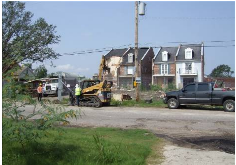
Fourteen properties on the 17th Street Canal are being demolished to allow for new levee and new stability berm construction. (USACE Photo by Kim Powell)
