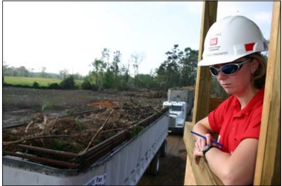
55 million cubic tons of debris have been removed by the Corps of Engineers in Louisiana and Mississippi - and work continues. (USACE Photo)
