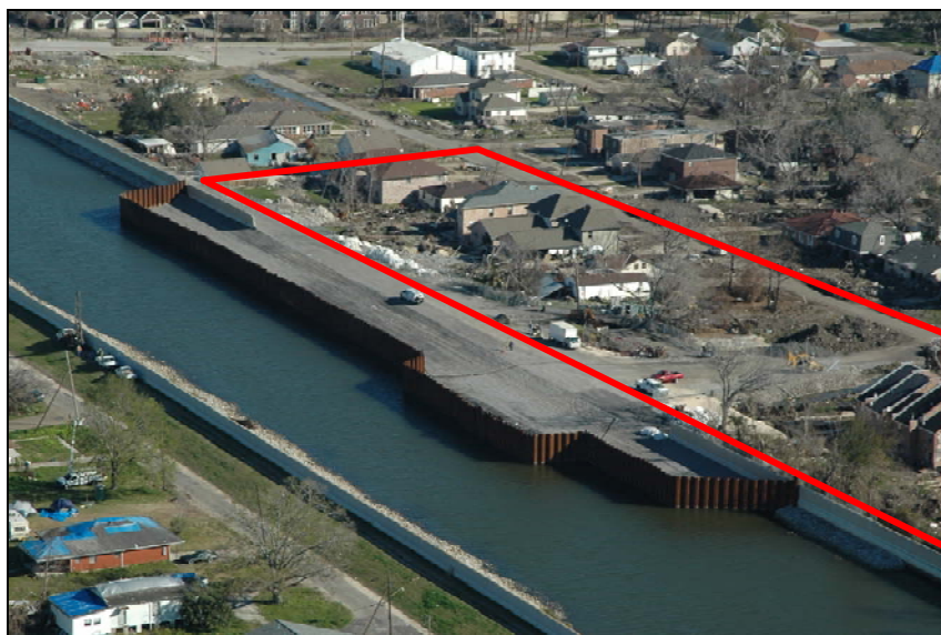
This illustration shows the area marked for demolition at the 17th Street Canal. (USACE Illustration by Erich Soraghan)
