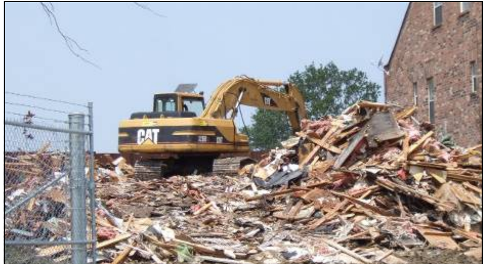
On August 9, Corps of Engineers' contractors began removing structures at 17th Street Canal so levee repairs can proceed. (USACE Photo by Kim Powell)
