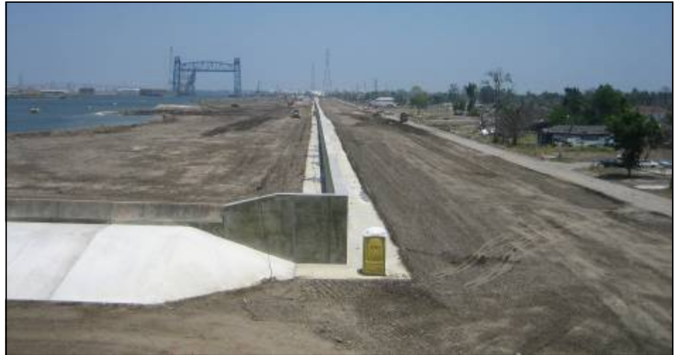
Floodwall at Inner Harbor Navigation Canal was completed on June 1, start of the hurricane season. (USACE photo by Paul Floro)
