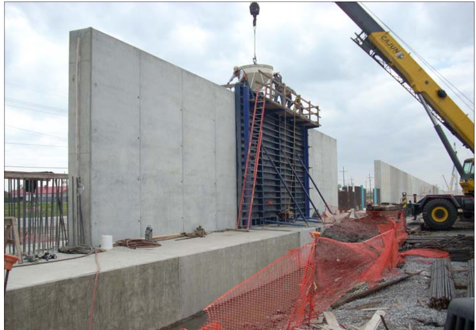
A new floodwall under construction at the Harvey Canal on the West Bank. At 15-19 feet tall, a 5-foot base slab, and pilings as deep as a 12-story building, this is one of the tallest and strongest floodwalls in the system. (USACE Photo)
